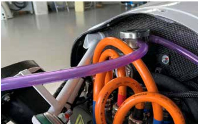
Figure 12-001 Hose connected to the expansion tank overflow port through a ball valve.
