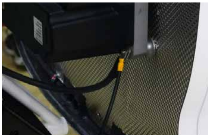
Figure 72-004 Grounding cables on power controller
