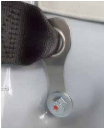
Figure 53-002 Safety harness attachment point on the cabin floor
