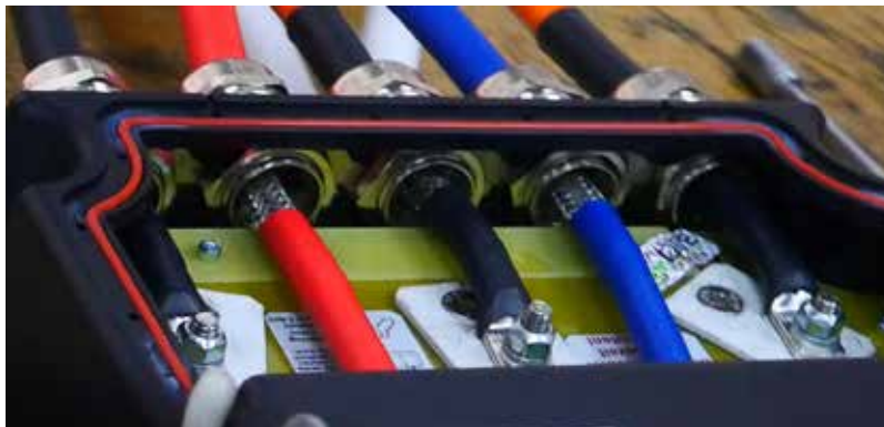
Figure 71-003 Power controller terminals
